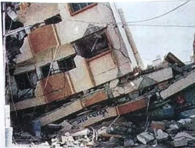
Damage caused by an earthquake
